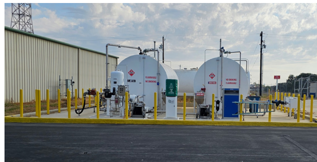
New 12,000-gallon fuel tanks at Pleasanton Municipal Airport.
