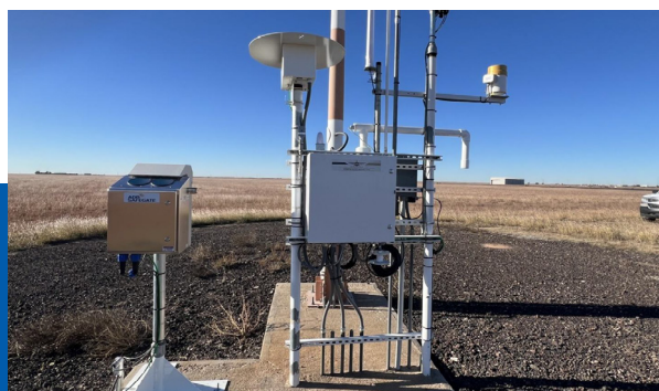
AWOS upgrades at the Moore County Airport.
